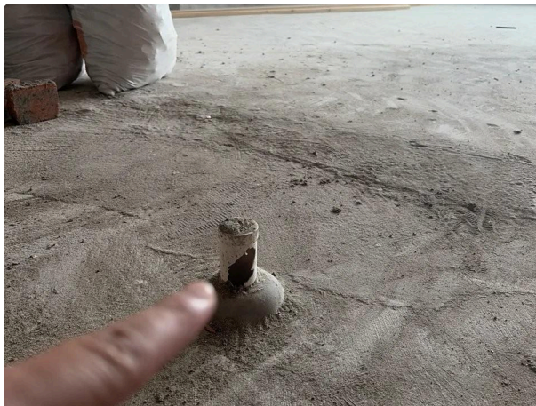
下水管破损未封堵
